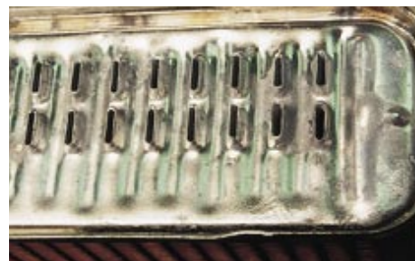
Well Maintained Cooling System
